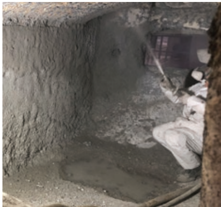
The repair is showing no signs of wear or spalling after 3 months service.
