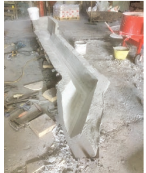
The launder remains in excellent condition after 2 months service.
